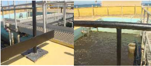
Figure 3. WWT Phase 1 complex of the GP1/ Z
